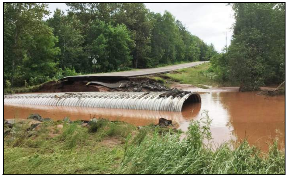
2016 ROAD FAILURE IN WISCONSIN
