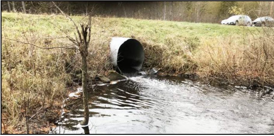
BEFORE: MCDONALD CREEK WITH UNDERSIZED AND PERCHED CULVERT The previous undersized and perched culvert over McDonald Creek had created a full aquatic organism passage barrier.
