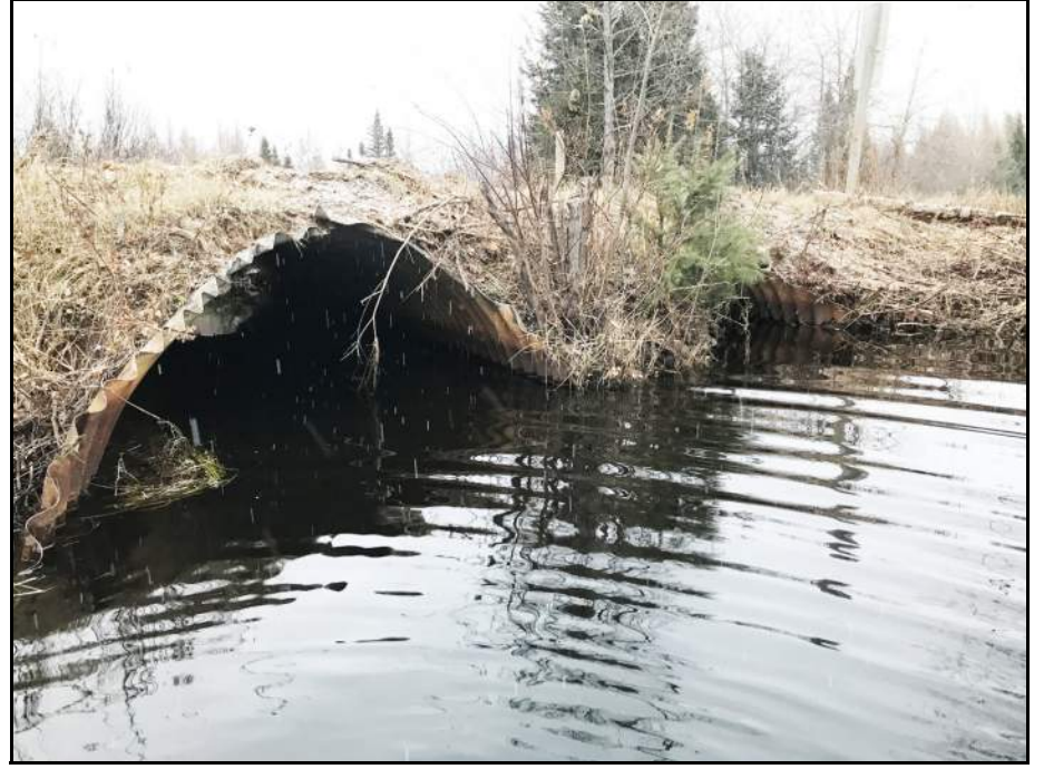
BEFORE: NO PASSAGE THROUGH THESE KINGSTONE CREEK CULVERTS Two undersized culverts created an aquatic organism passage barrier on Kingstone Creek.
