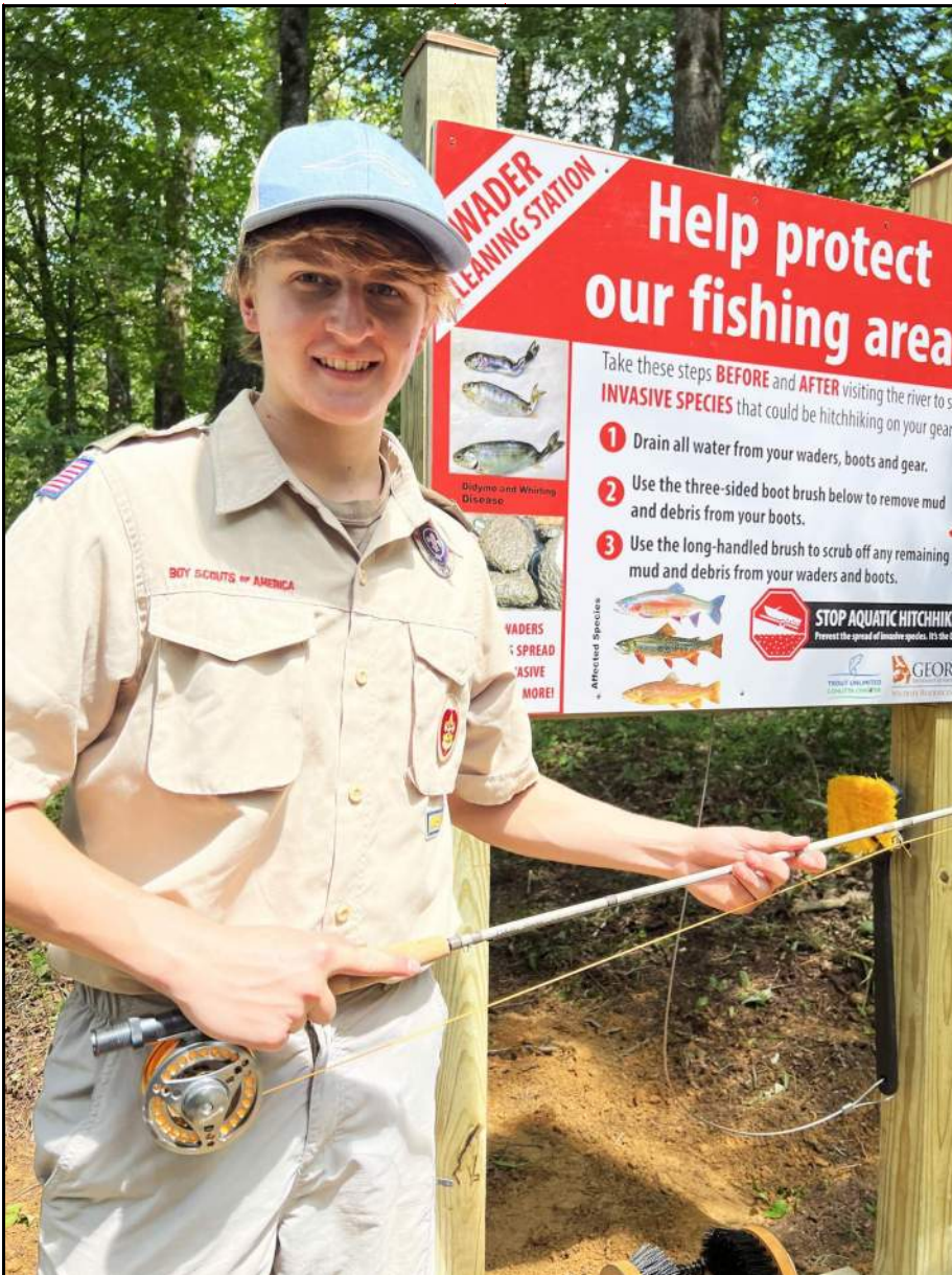
SCOUT CREATES WADER WASH STATIONS IN GEORGIA Noah Ottinger spearheaded an effort in Georgia to build wader wash stations to protect his favorite trout streams.
