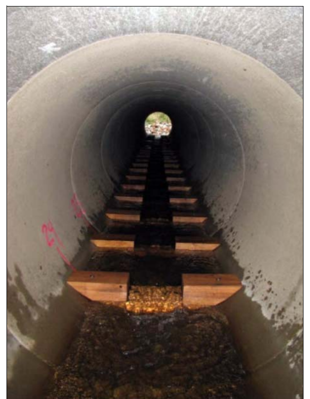
BAFFLES HOLD WATER FOR TROUT PASSAGE Wooden baffles installed inside the 62-foot-long culvert on Getchell Creek now allow for trout passage under Hwy. 55 in Langlade County.
