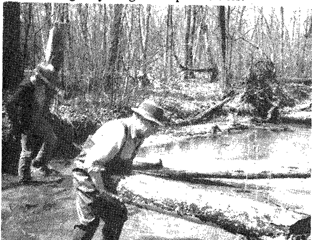
"It's a good thing this timber is so light - must be a balsawood forest". Deadfall removal was critical to reduce bank erosion. Bob Burnham shows how it's done.
