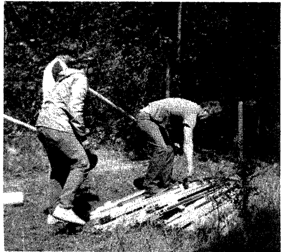
Roger Denil, Bob Solboe, and Dale Druckery select metal stakes for lining up fence rows.
