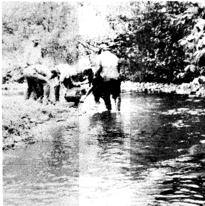
Members of the Green Bay Chapter installing bank cover structures on the First South Branch of the Oconto River near Mountain, WI.
