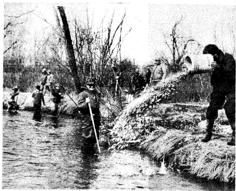
40 yards of gravel were spread on Rocky Run Creek to create a spawning area for trout.
