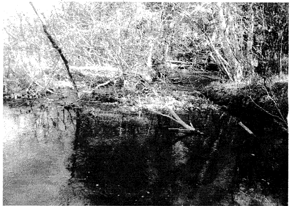
Dalton Creek below Hwy. 64 (Langlade Co.) where gravel piled up in stream after culvert washed out
