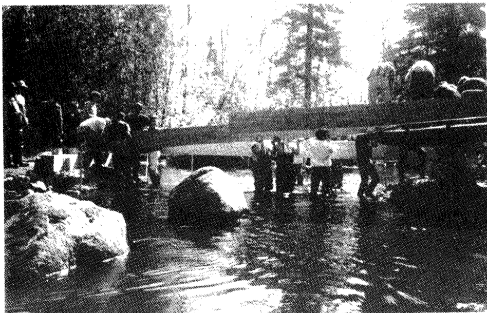
Bridge being built over South Fork Thunder River. Large boulders placed in stream to prevent ORV's from crossing stream.
