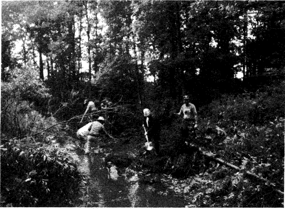
T.U. members from Green Bay, Lakeshore and S.E. Wisconsin chapters prepare bank of Ben Nutt Creek for sodding.
