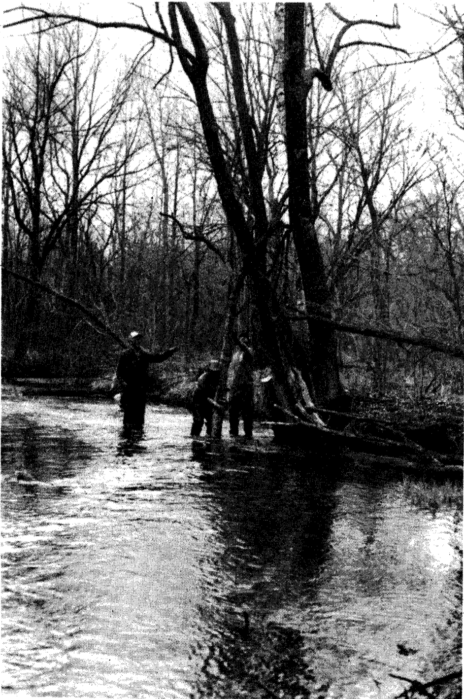
Central Wisconsin Chapter members building brush bundle deflector on the west branch of the White River (Waushara County).
