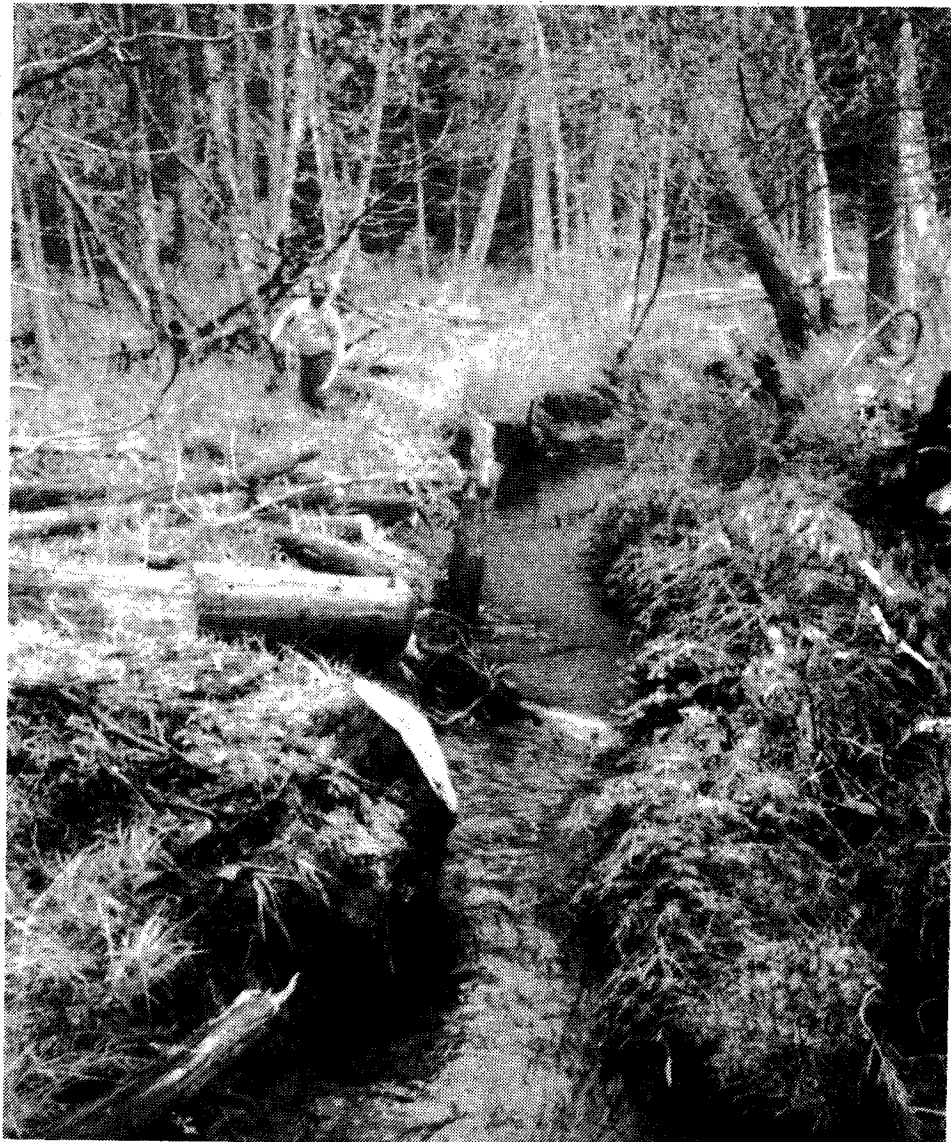
Brush bundles placed along Brehmer Creek will trap silt and deepen stream channel.
